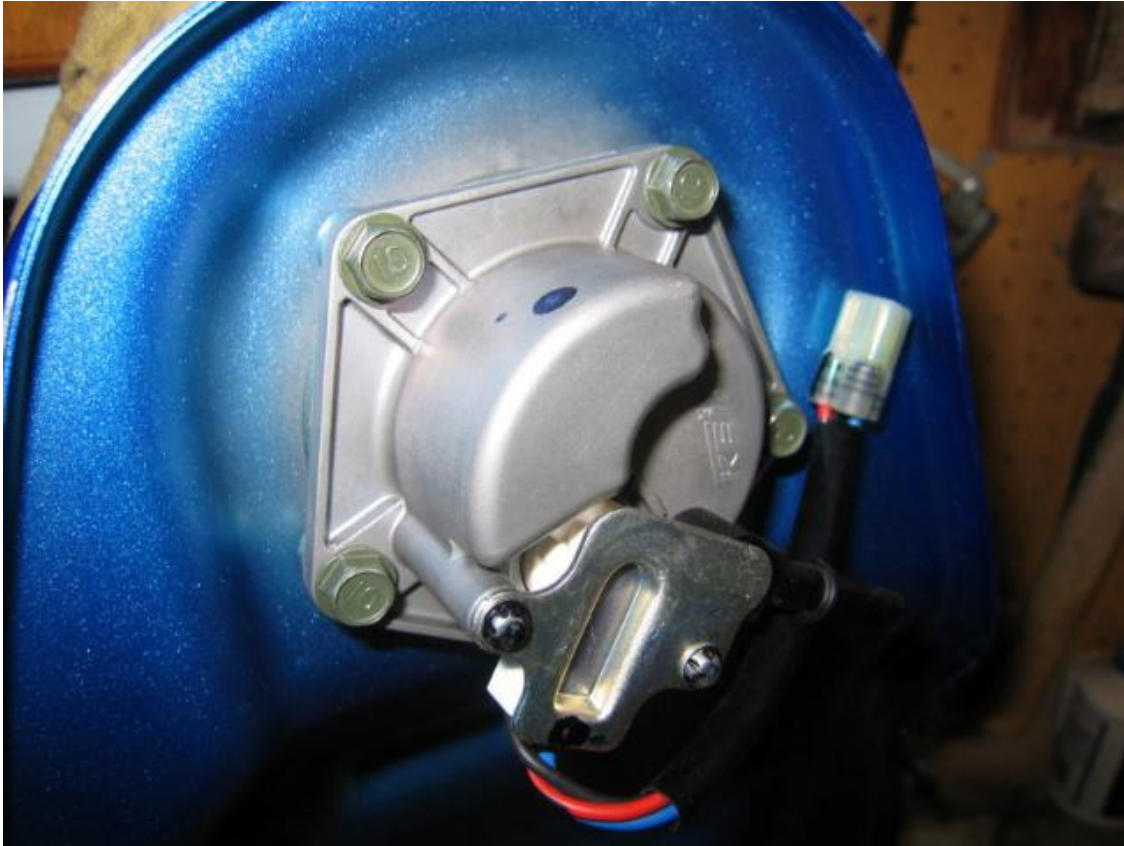
Tank with pump
